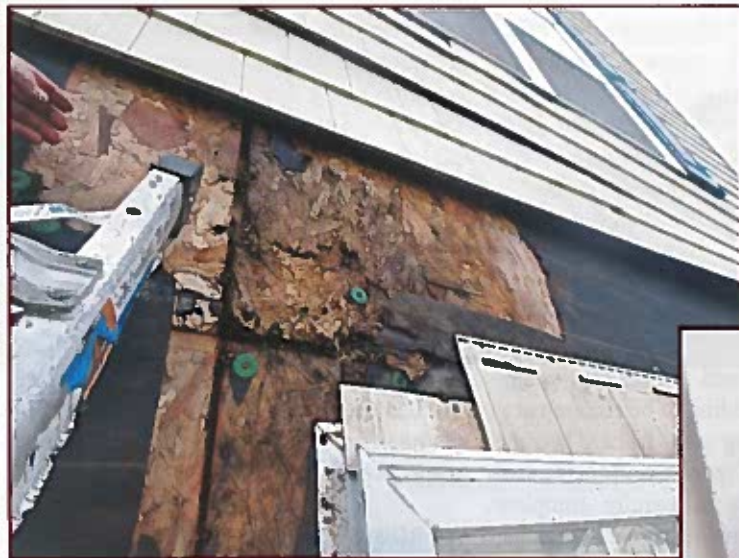
Figure 2 – Exterior wall water damage.
