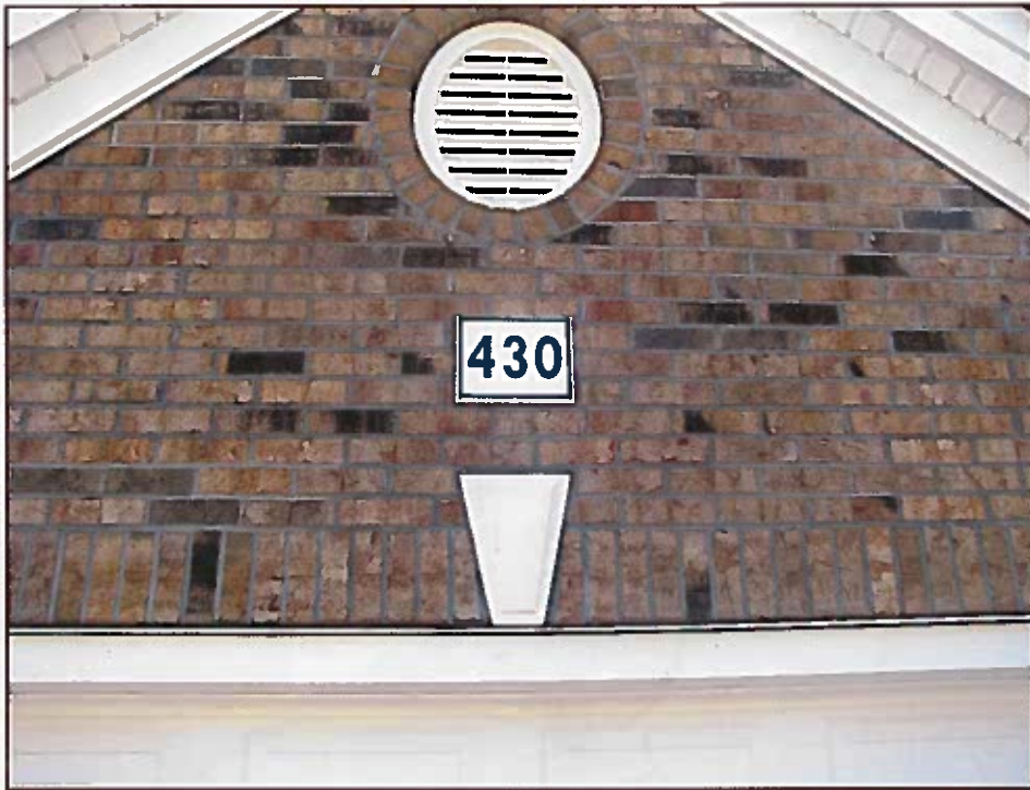
Figure 1 – Absence of weepholes above a garage opening in brick veneer.
