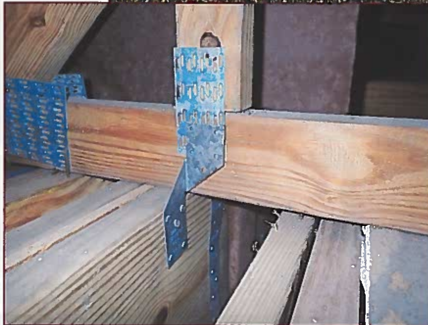
Figure 6 – Missing truss hold-down fasteners.
