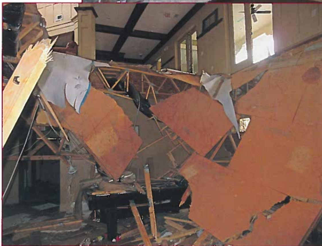
Figure 3 – View of collapsed floor framing.
