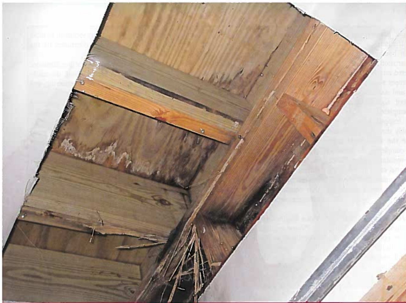
Figure 6 – View of water damage at balcony.
