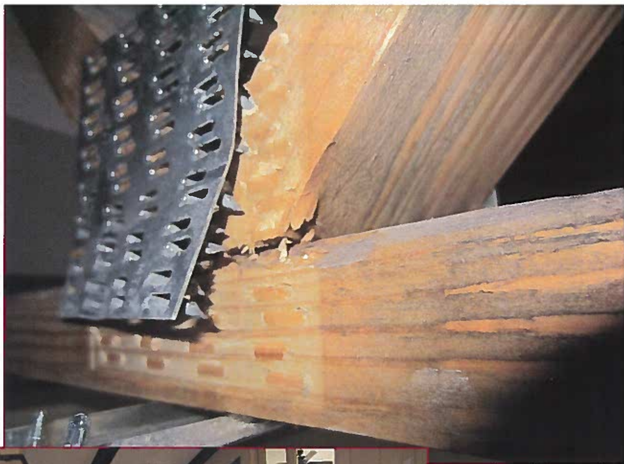
Figure 2 – View of damaged wood truss due to dynamic condition.
